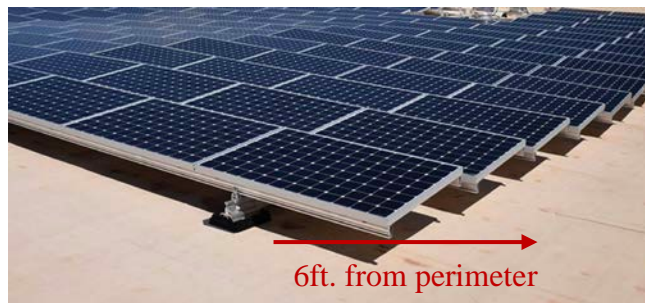
Figure 1.4: International Fire Code requires a minimum of 6ft perimeter around the edges of a roof.
