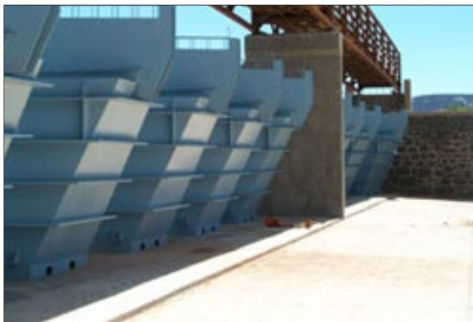
Fusegates Installed at the Black Rock Dam. Fusegates are adjustable gates that can “increase both spillway capacity and reservoir storage” at a lower cost than heightening a dam (Afshar and Takbiri 2009; Falvey and Treille 1995:512). Photo source: Gannett Fleming (2002); reproduced with the permission of Gannett Fleming, Inc.
